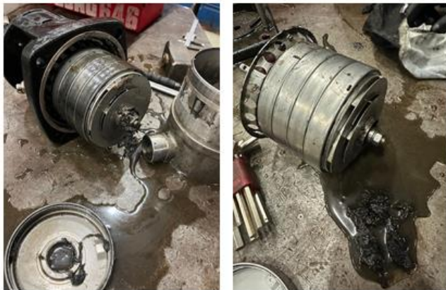
Clogged pump and valve 27/11/2024
