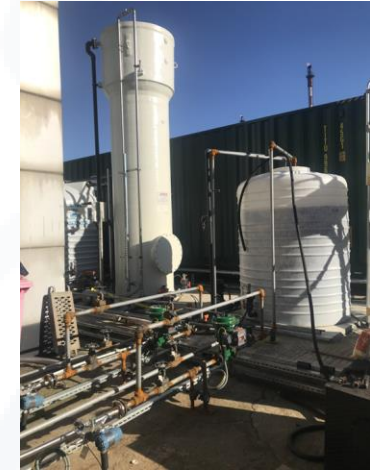
GRANULAR BIOLOGICAL REACTOR
