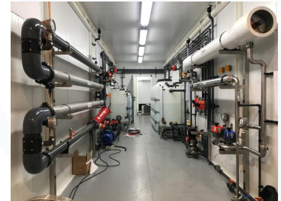
ULTRAFILTRATION + REVERSE OSMOSIS (REGENERATED MEMBRANES)
